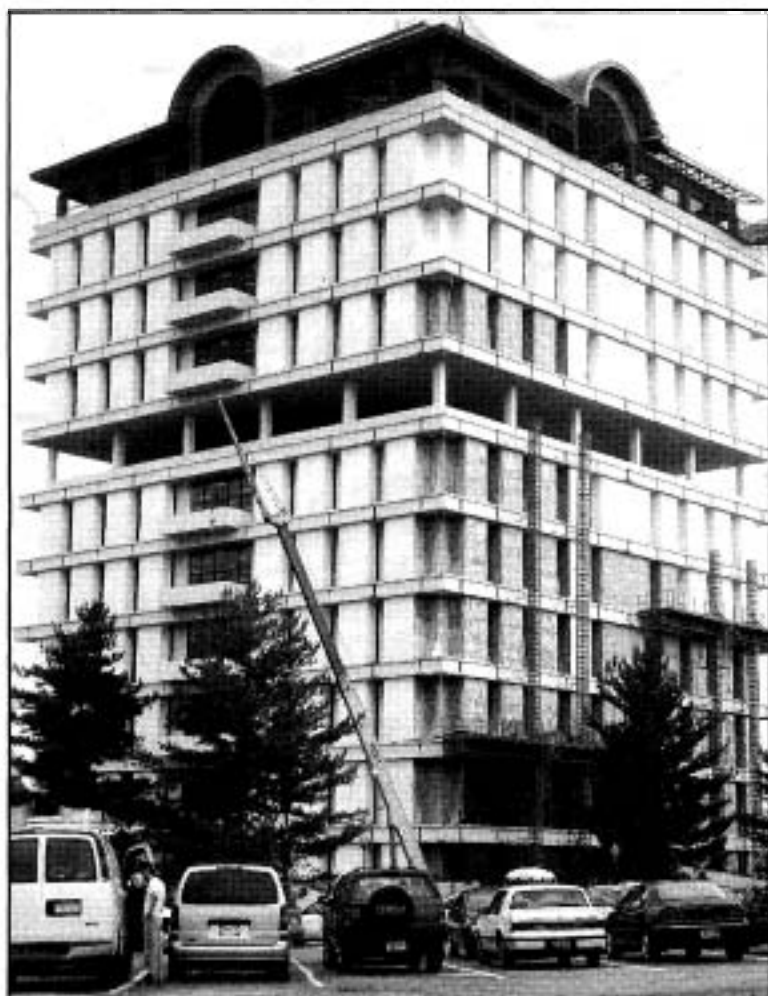
The Chanticleer/Cafe Williams Construction workers remove marble slabs from the exterior of Houston Cole Library, replacing them with darker granite slabs.
