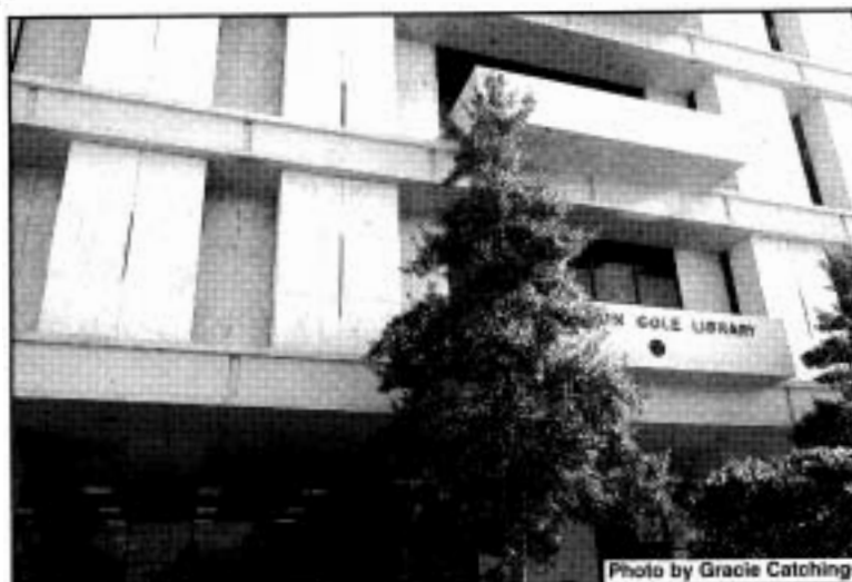
On close examination, the cracks in the Houston Cole Library become evident. Renovation is tentatively set for this summer
