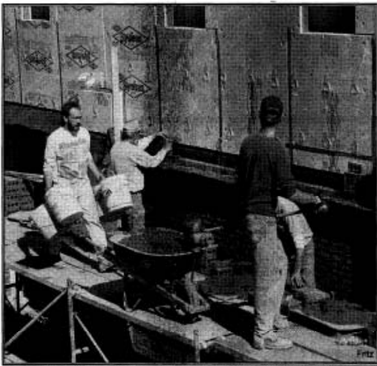
The brick facade on west side of the Theron Montgomery Student Commons began to take shape beginning on Monday of this week. Also, concrete wheelchairs are completed on the south first floor entrance (basement), as part of the on-going renovations.
