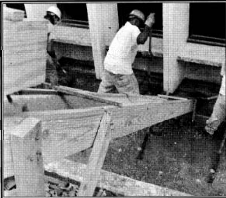
Work continues on the Thruout Montgomery Student Commons Building, as crews begin pouring fresh cement footings around the base of the TMB last week.
