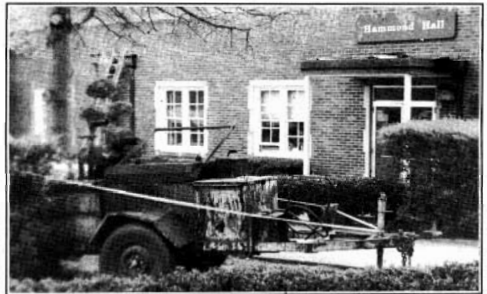
Last week, workmen began renovating Hammond Hall, which is the home of JSU's art department and art gallery. The University is also planning additional campus renovations. Tamara Miles
