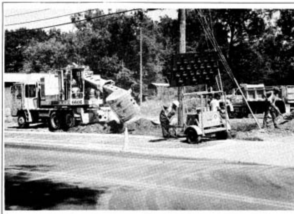
Highway work: Dangerous intersections, like the one at Mountain street, receive repairs
