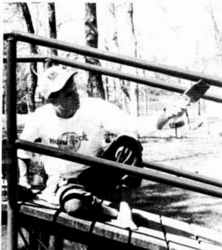
Stephen Johnson repaints a bridge in Germana Springs Park as part of a service project for Alpha Phi Omega.
