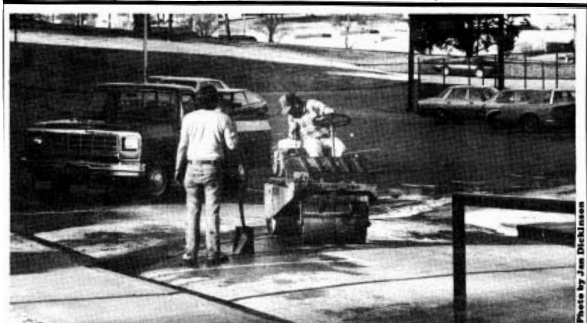
Most of the trenches on campus have been covered up due to complaints
