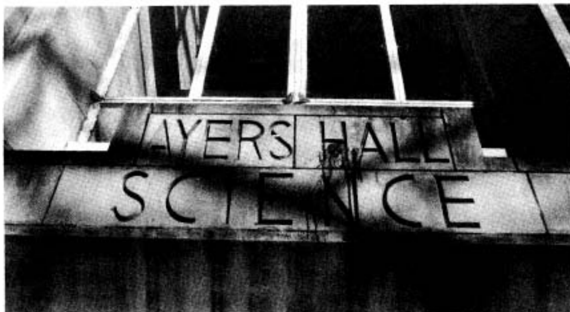
Above: Entrance to Ayers Hall shows sign of damage
