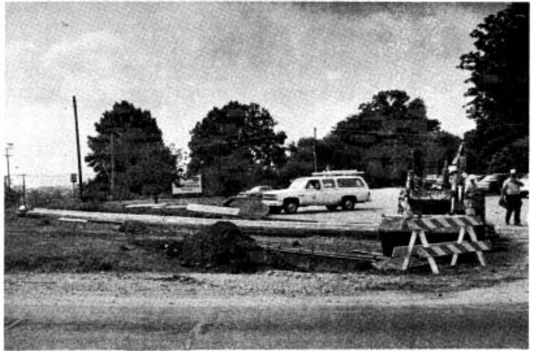
Work continues at corner of Hy. 204 and Pelham for new turning lane.
