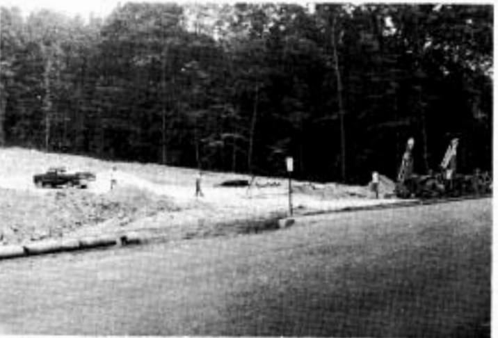
The felling of trees has leveled the corner at Bennett Drive and Church Street opposite Rowe Hall. The unloading of tons of fill dirt and the laying of enormous pipes to direct drainage are only two steps necessary for adding yet another parking lot.
