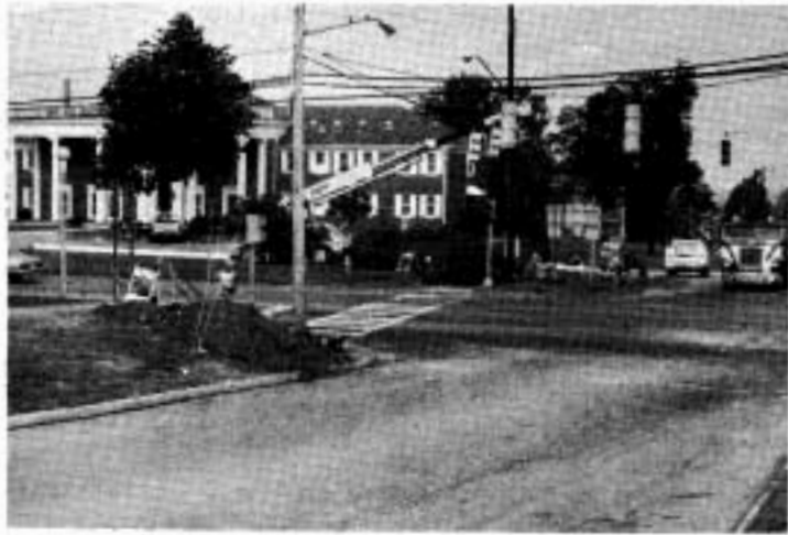
Mounds of red clay on the corners of Nisbet Road and Bennett Drive signify installation of a new steamline intended to reduce the fuel bill for the University by winter '83-'84.
