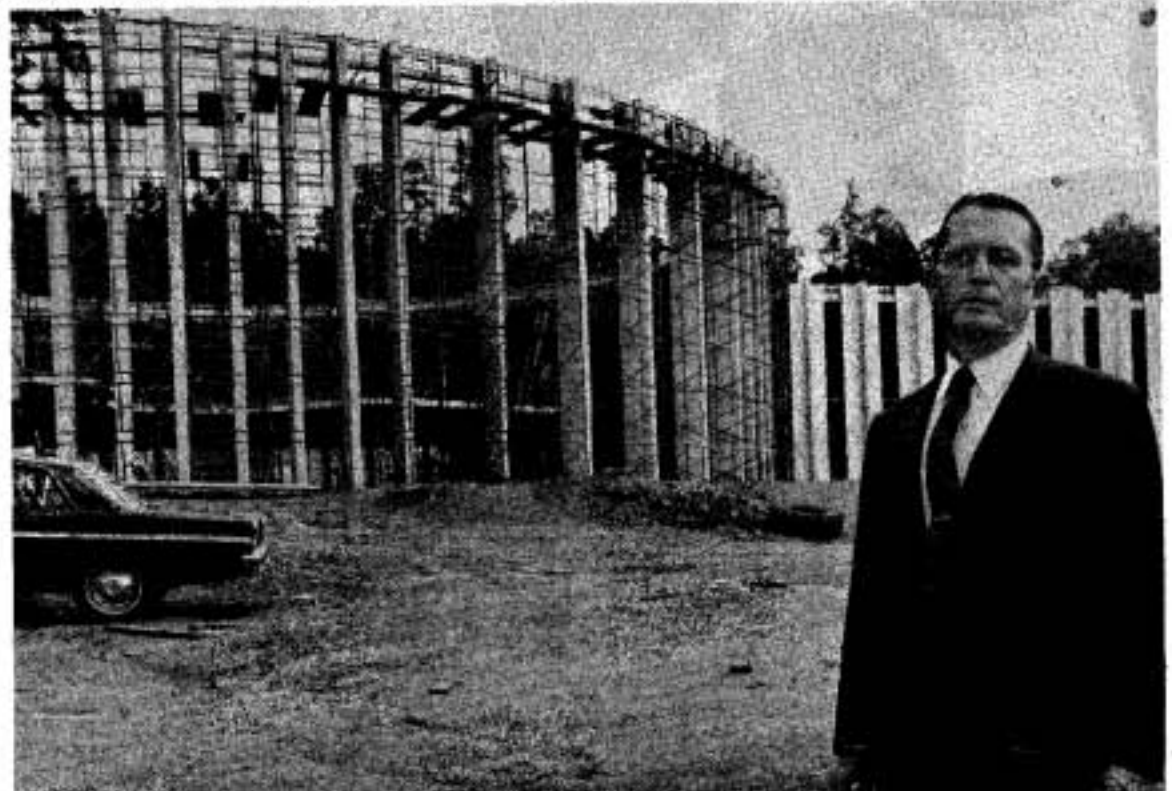
Rep. Hugh Merrill of Anniston stands in front of the partially completed business administration building which will bear his name. The $1.5 million structure will be completed in January.
