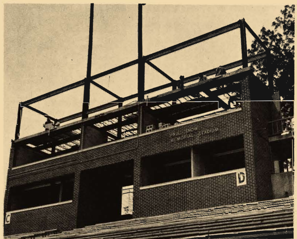
NEW ADDITION TO PRESS BOX -- Additions to the pressbox at Paul Snow Memorial Stadium will be completed this summer. An new story is being added on top to accomodate sports writers covering the Gamecocks.
