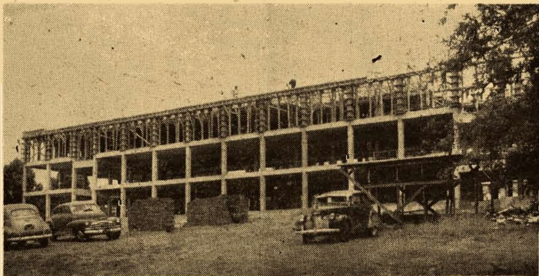
SIGNS OF PROGRESS—Sure signs of progress on our campus are the new 150-bed wing now being built as an addition to Pannell Hall and the proposed science building, to be located on the north side of the campus, just east of the International House. The new dormitory addition is expected to be finished some time during the second semester, and the contract for the science building will be let on Sept. 21.
